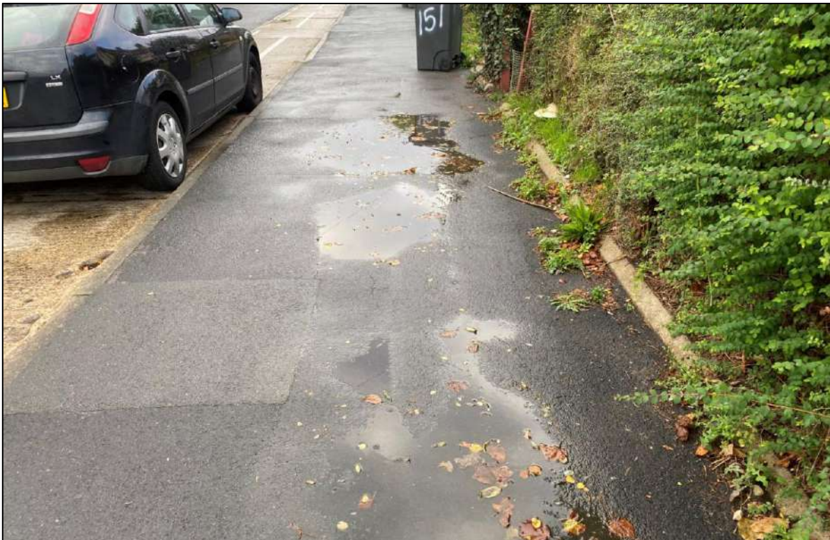
Image 16: Ponding on Footway
