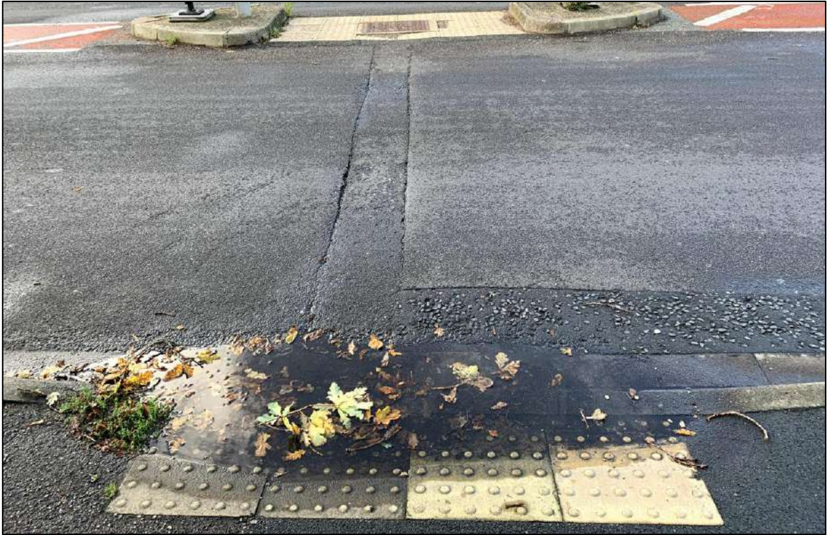
Image 15: Ponding Across Pedestrian Crossing on Wych Lane
